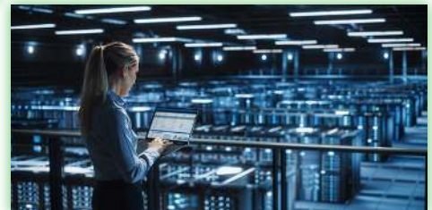
Micro Data Center and Server Room
